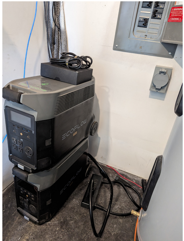
EcoFlow units placed near 240V outlet that ties into breaker
